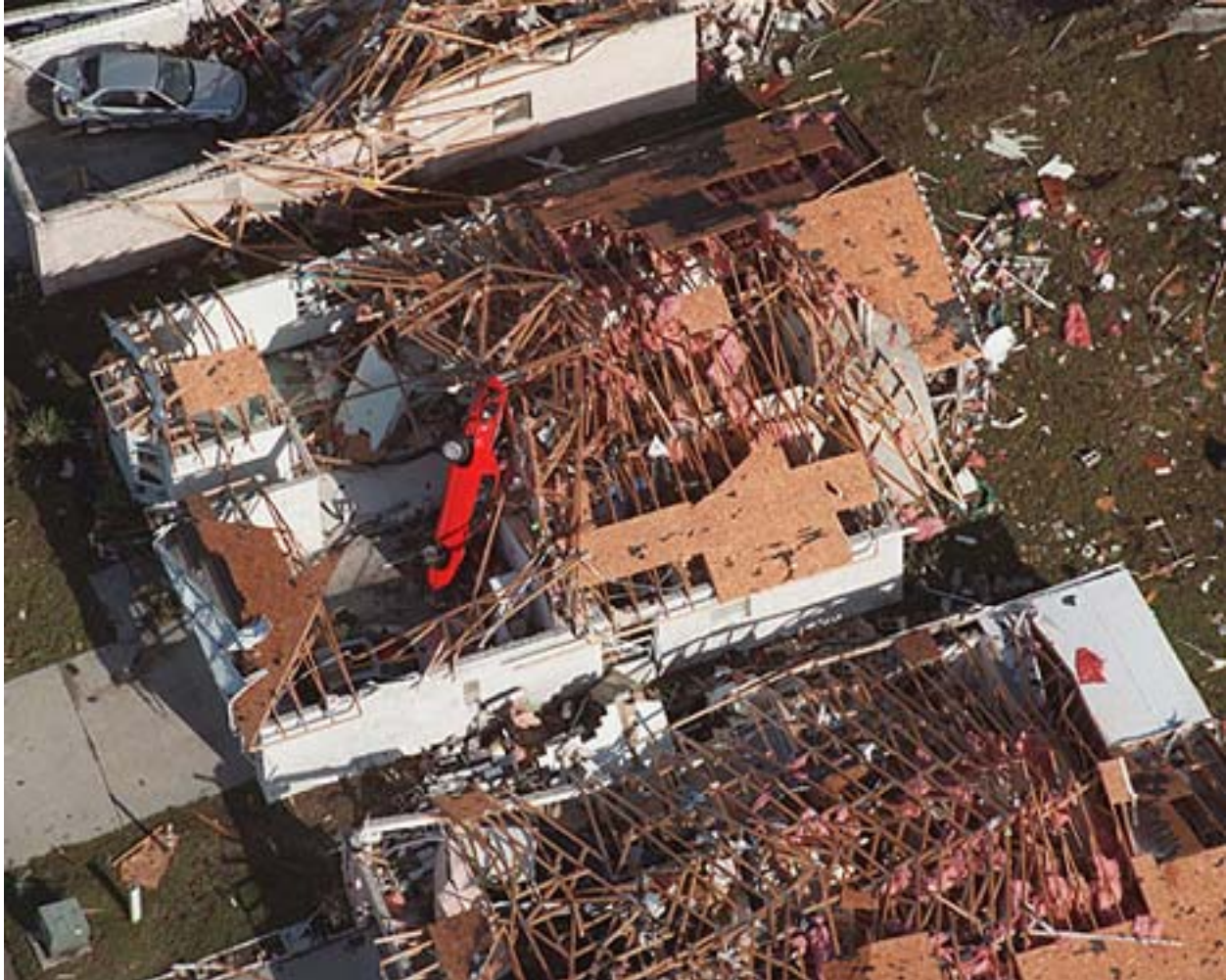
Figure 2. Damaged Osceola County home with a car resting inside its walls (Red Huber, The Orlando Sentinel).
